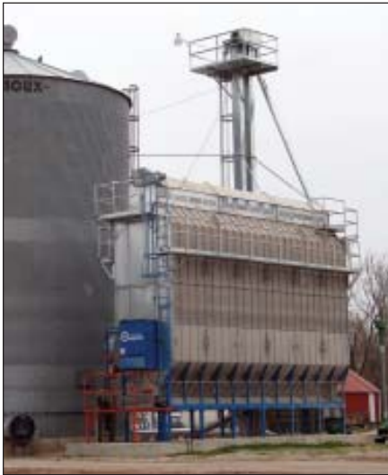
New 1,500-bph Delux DPXSL continuous flow dryer installed at Browns Valley Community Elevator in Browns Valley, MN provides the cooperative with higher drying capacity and lower noise levels. Photo courtesy of Delux Mfg. Co.
